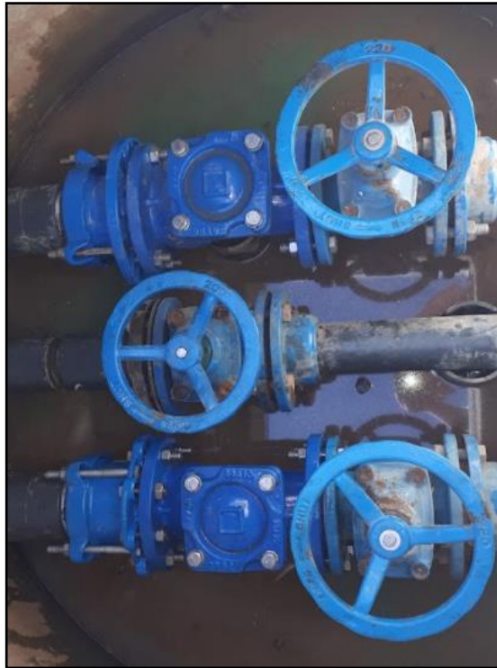
Clapet P2 PR Clos Lagarde
